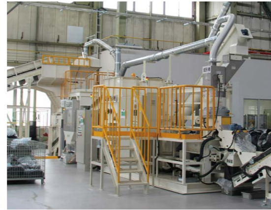
RPF production equipment (Kurobe Ekko Plant)
