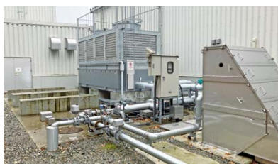
Cooling unit at the Namerikawa Plant
