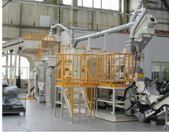
RPF production equipment (Kurobe Ekko Plant)
