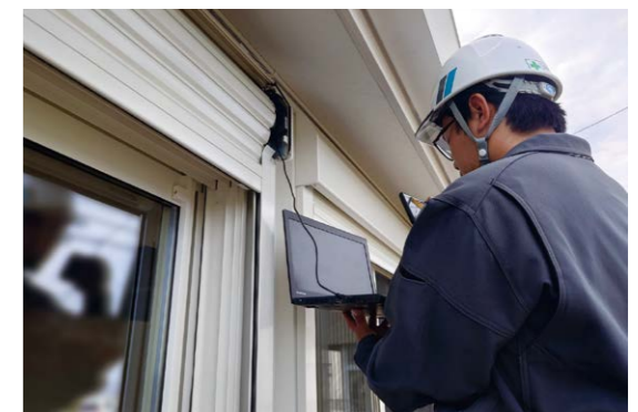
Maintenance of electric equipment using digital tools
