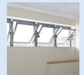
Natural ventilation windows (Balance Way) The grid itself is balanced to provide efficient ventilation.
